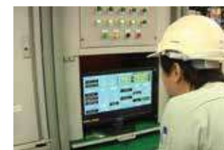
Control panel (Singapore factory)
