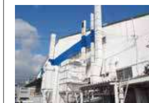
Ventilation equipment (Shiga factory)
