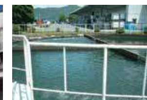
Effluent treatment facility (Kyushu factory)
