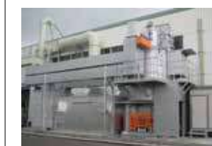
Deodorizing equipment (Kyushu factory)
